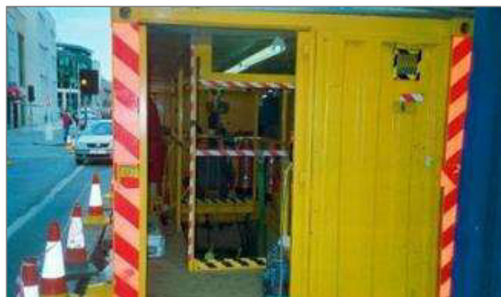
Figure 13: HV cable jointing container
